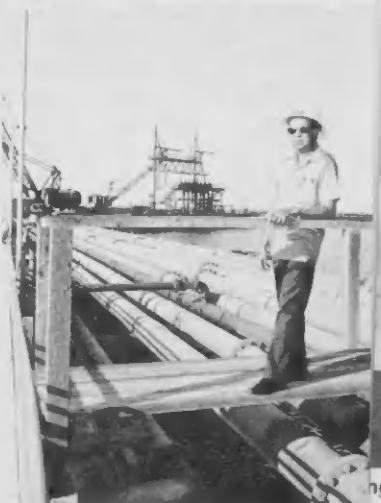
Night Shift Coordinator Adrian stands over pipe banks. Night Shift Coordinator Adrian ta aki ariba linja di tuberla
